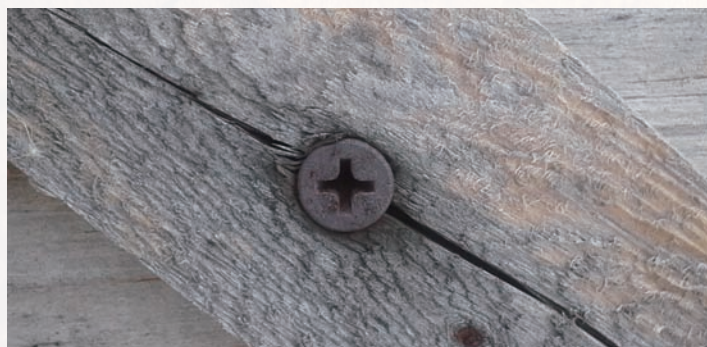
Figure 1: Zinc Plated Fastener Example in Alternate Treated Lumber After Several Years Exposure
